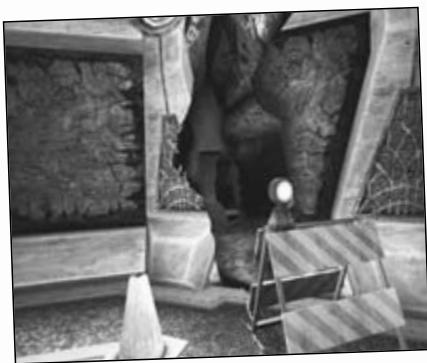
Crack in hallway wall revealed rotating wall, which had a gap in it.
