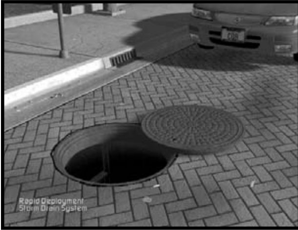
Fig. 15-1. The Los Angeles storm drains.
