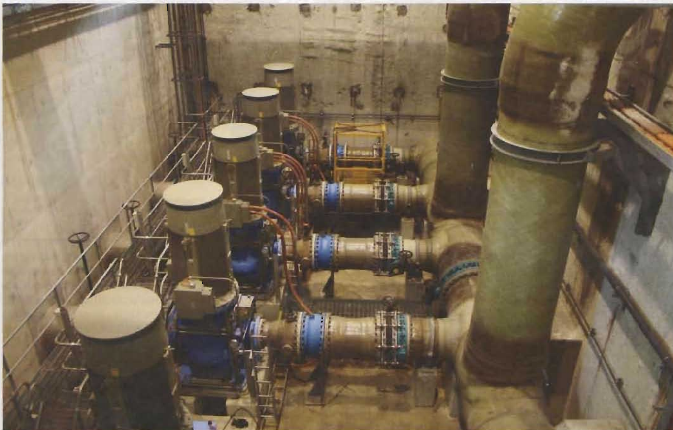
This installation uses six high pressure centrifugal pumps drawing 2600kW each and pumping 1144 cubic metres/hour. They are made from super duplex stainless steel and need to be very well balanced during installation. Manufacturer was Clyde Pumps in Scotland. (courtesy Water Corporation)
