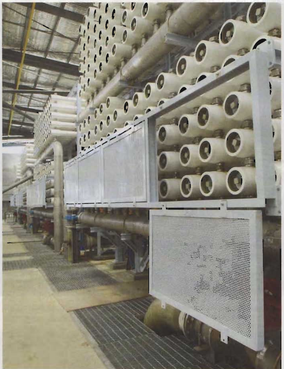
Reverse Osmosis pressure vessels. Each contains seven reverse osmosis membranes tightly wound in coils. The pressure used to force the water through the membranes is very high, up to 1000 psi. At this pressure salt water is very corrosive so high quality stainless steel is used (courtesy Water Corporation WA).
