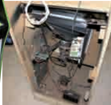
» Found with no back door and exposed mains cables.
