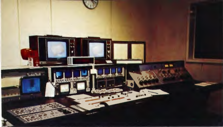
Master Control Room.
