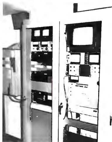
Satellite Earth Station operated by TV-11 is mounted on an adjoining parking garage roof. System uses an 11-meter Steerable Receiving Antenna and provides access to TV newscasts originated by ITNA-affiliated stations. Rack equipment for the Earth Station is conveniently located in the Technical Area near Master Control.
