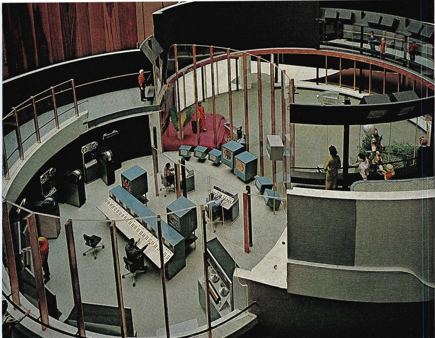
All of the control equipment is grouped in this area. The equipment room is under the ramp at left.
