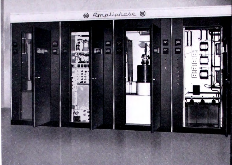
FIG. 2. Easy access to all tubes and tuning controls is through the front doors. The cubicle on far right contains the new silicon rectifiers, next is one of the PA stages. On the far left the other PA stage and next to it the exciter and driver stages.
