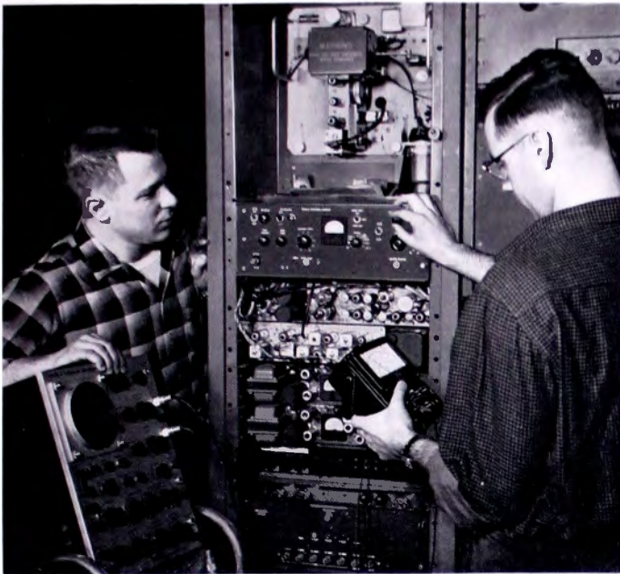
FIG. 5. Transmitter operators, Wilfred Mank (right) and John Jacobsen (left), perform routine maintenance on the TVM-1A Microwave equipment that brings the WMTW signal to the transmitter from the Poland Springs Studios 50 miles away.
