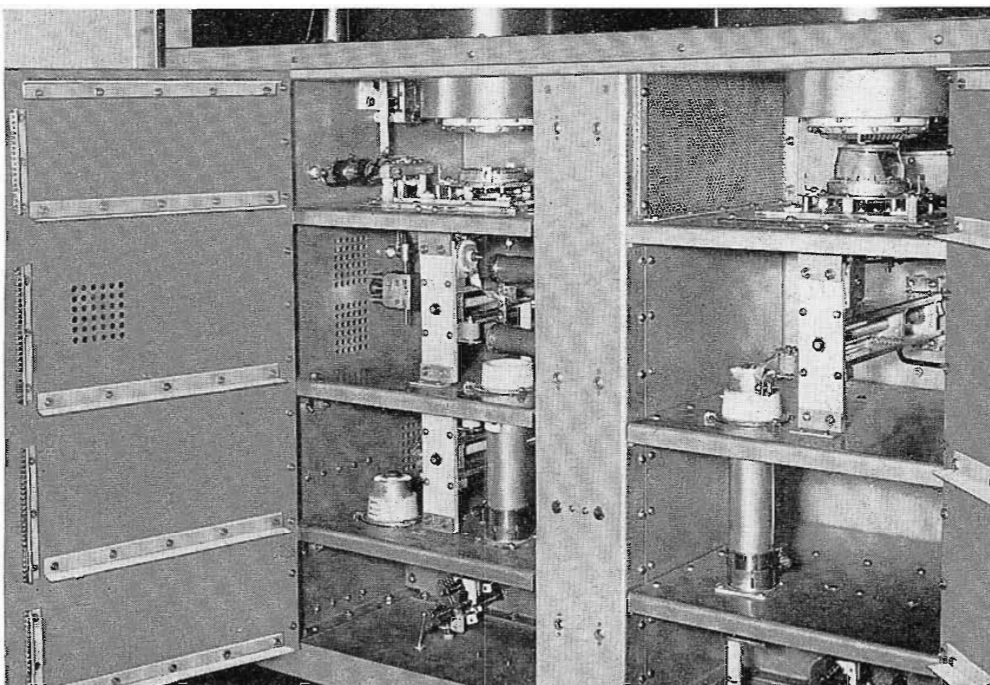
FIG. 5. This is the R-F Driver unit. The visual driver is shown on the left and the aural on the right. With panels open note ease of accessibility.
