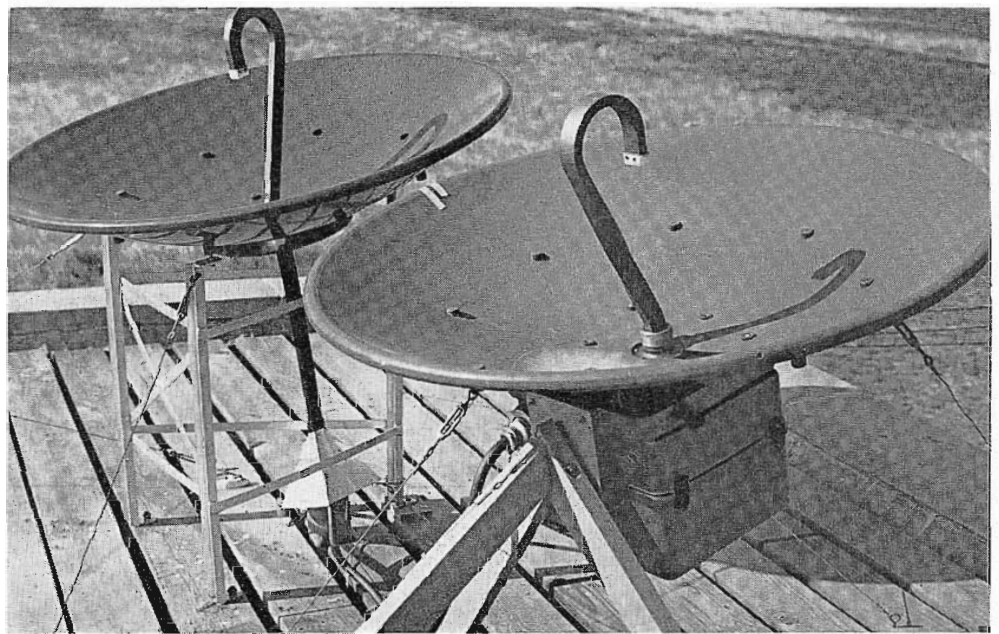
FIG. 24. (Left) STL link waveguide feeds directly through roof into video racks beneath. (Right) Remote pick-up microwave unit, placed on roof as STL standby when not in use for remote work.
