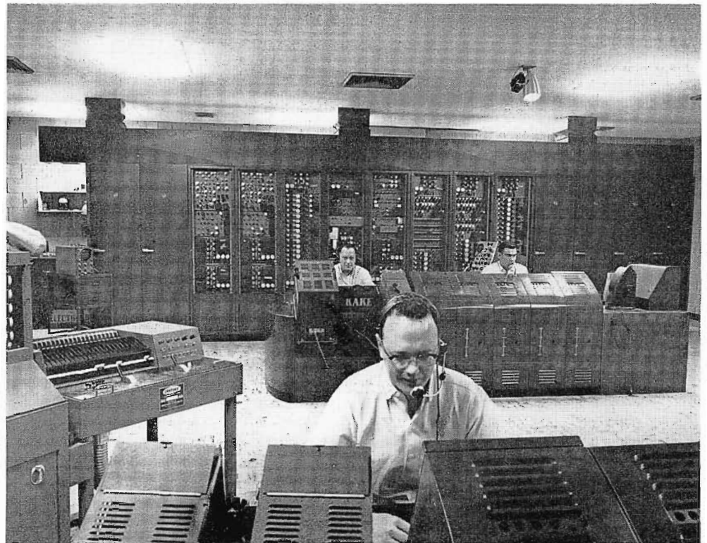
FIG. 15. Rack equipment behind master control: terminal equipment for audio and video; stabilizing and distribution amplifiers; and power supplies.
