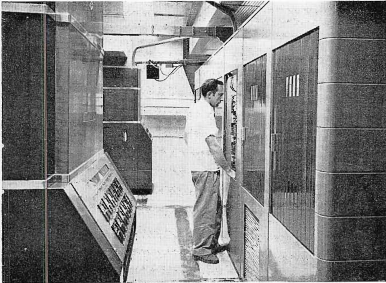
FIG. 29. Rear view of transmitter cubicles. At left, are 50-kw power amplifiers. Note generous aisle area.
