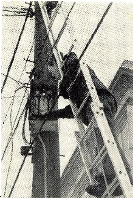
Fig. 7. Lineman completes wiring of ADO-10 box during the installation. Each antenna distribution box feeds 10 connections and the units can be connected in series to feed an almost unlimited number of receivers.
