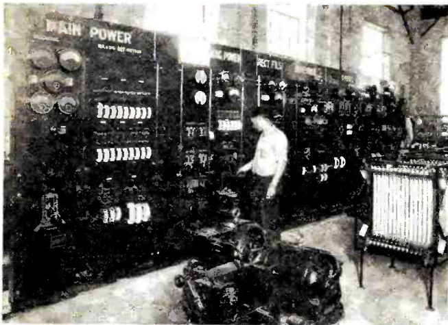
This is a close-up view of the control panels of the Marconi beam system at Rocky Point
