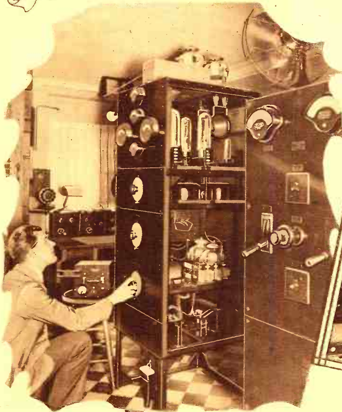
THE TRANSMITTER AND CONTROL PANELS. In the transmitter can be seen the large tubes and tuning apparatus and on the right is the panel on which is mounted the apparatus which controls the motor generator set.
