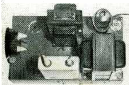
This power supply puts out 500 volts at 200 ma, with choke input. The meter measures the output current and the small lamp, in the centertap, is a fuse.
