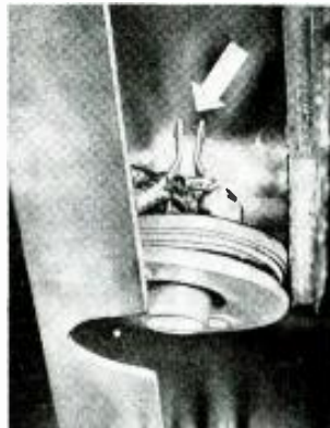
One of the Pittsburgh BBB's faulty circuits.
