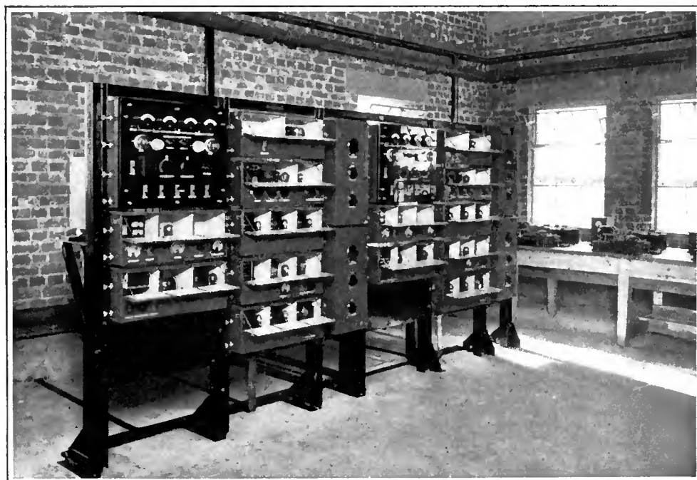
RECEIVING EQUIPMENT AT THE BRIDGEWATER STATION
