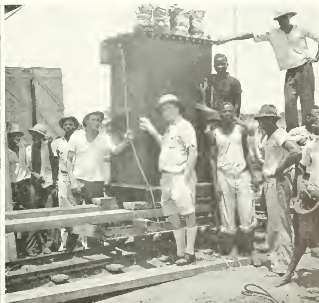
ENGINEER BROWN GETS THE HELP OF NATIVES IN PUTTING INTO POSITION THE HUGE TRANSFORMER, WHICH WAS PART OF THE RCA TRANSMITTER INSTALLATION AT BRAZZAVILLE. NO CRANES OR DERRICKS WERE AVAILABLE.
