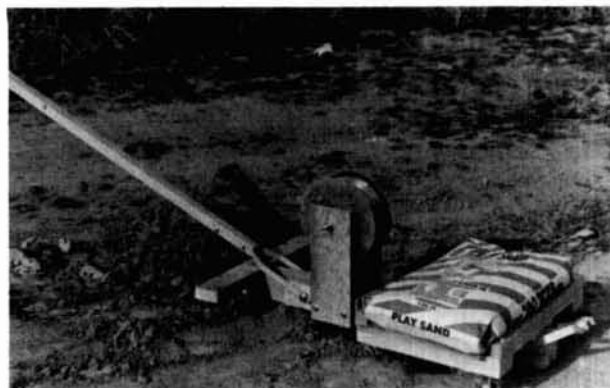
fig. 4. Wire plow in position over starting hole. Handle guides plow; 100-pound sandbag provides necessary weight.
