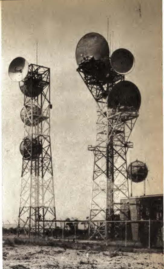
The repeater station at Madden's Plains, south of Sydney, is typical of similar broadband repeaters all over Australia. These must be capable of handling the more complex signals when colour TV is introduced.
