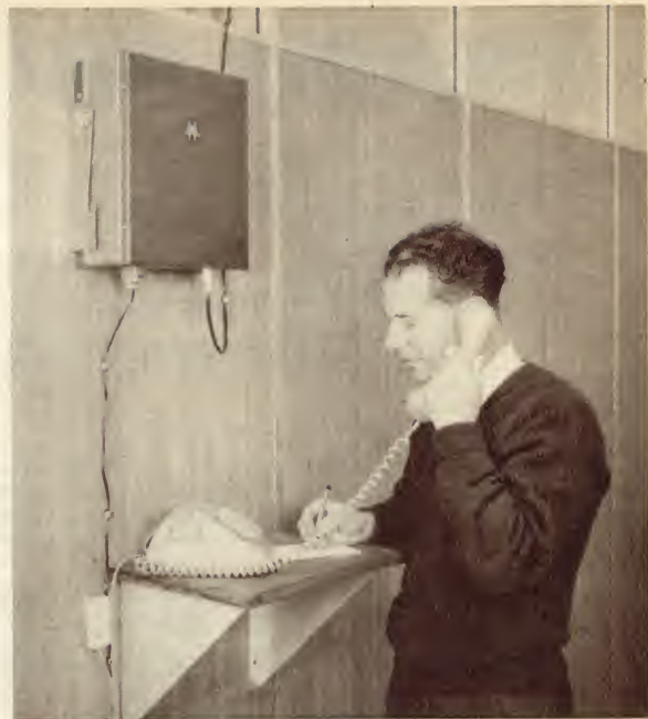
A subscriber's terminal installation
