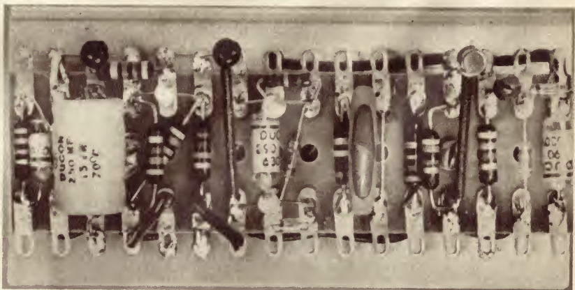
The reverse side of the assembly, this board contains the noise amplifier at the left, followed by the phase-splitter, detector and pulse amplifier at the right. This should be studied with the wiring diagram on page 81.
