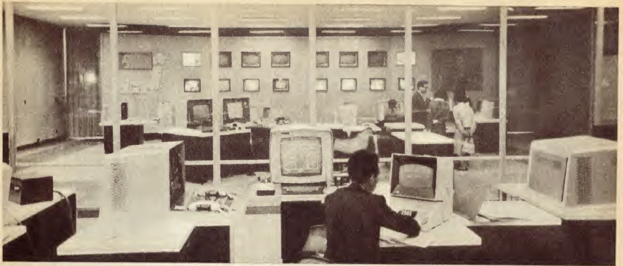
Broadcasting control centre of NHK's five network complex, where TOPICS is installed.
