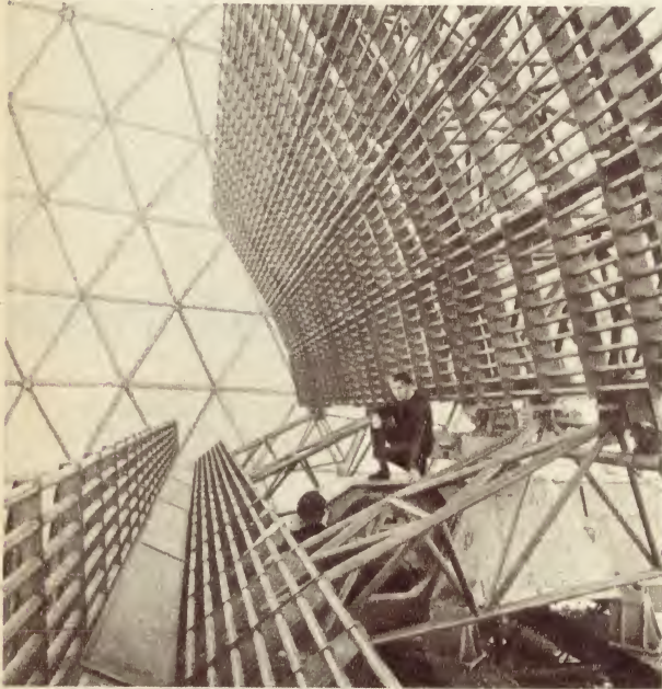
Nearing completion on Lowther Hill, in Southern Scotland, is this Marconi radar which will give added coverage to busy air routes near Glasgow. Rising above the aerial turning gear is the parabolic reflector, and on the left of the picture is the linear wave-guide feed extending the full 52-foot length of the aerial. The triangular configuration in the background is part of the geodetic radome to give the installation complete weather protection.
