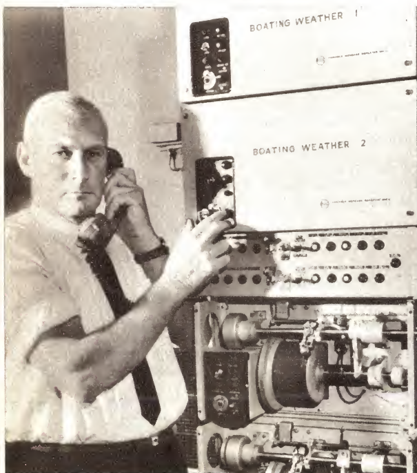
Supervising technician Graham Trundwell checks Rola Variable Message Repeater units in use at the G.P.O. building in Sydney.
