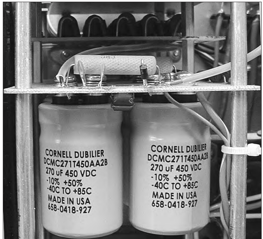
Fig 7.44 — Example of the filter capacitor/bleeder resistor installation in a high voltage power supply.
