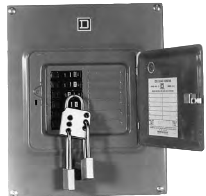
Fig 28.2 — If the switch box feeding power to your shack is equipped with a lock-out hole, use it. With a lock through the hole on the box, the power cannot be accidentally turned back on. (Photo courtesy of American ED-CO)
