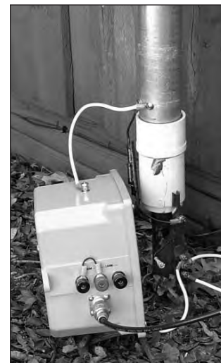
Fig 24.16 — The finished matching unit at the base of the author's 43-ft antenna (strapped for 80 meter operation).
